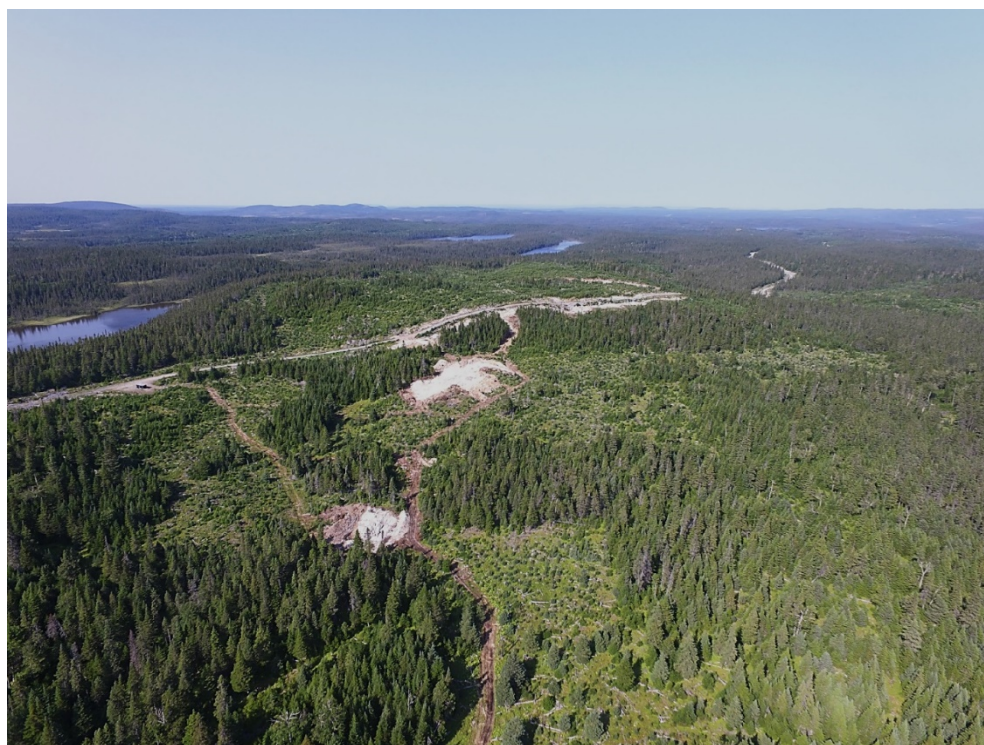
Figure 154: Sail Pond Project Area Access Road and Trenching at Heimdall Zone, looking north.
